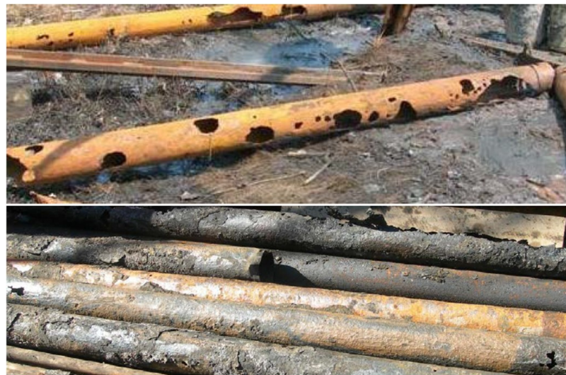
Figure 3. External steel casing corrosion from acidic water attack [32].
